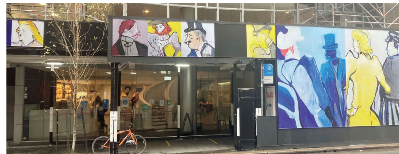
Jasper Knight Exhibition adorning the facade of AFS centre during renovation works.
